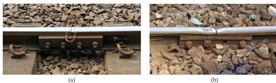
Figure 1. Two examples of rail joints: (a) Invisible damage: loose bolts and (b) visible damage: missing bolt and battered rail surface.
